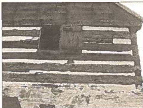
“milkhouse - in need of repair”
