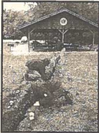
Top: PCC Crew Members, Jesse, Derek and Miriam complete the trench for a new powerline.
