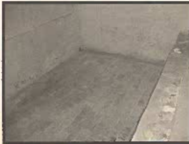
Floor of Milk House after repair by Renfrew Staff member, Ron Harbaugh.
