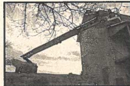
Renfrew's PCC crew used a Grove Man-Lift during the month of February to repair the gutter system on the Fahnestock House. They also painted the trim and side of the porch.
