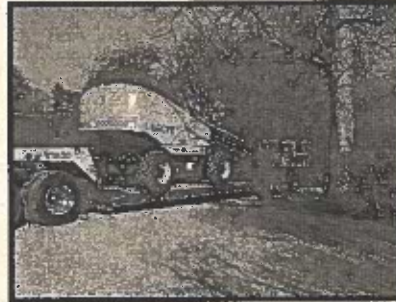
Grove Worldwide provided us with a Man-Lift for gutter work and painting on the Fahnestock House. The lift was brought to Renfrew by D. L. George & Sons and returned to Grove by D. A. Helman Excavating.
