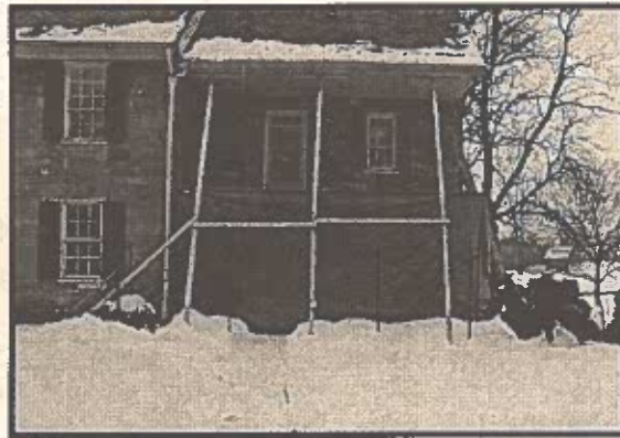
Renfrew’s front porch is currently undergoing a major renovation. The project is scheduled for completion this spring.
