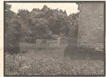
Picket fence constructed near the main entrance to the Fahnestock House. This is the first section of a fence that will ultimately line the hillside drop-off.
