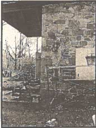
Richard Ressler repairs the pointing on the North side of Renfrew's Smoke House. Mr. Ressler spent over a week at Renfrew, repairing exterior areas of the Smoke House, Museum and Visitors Center Barn. He also tackled two of the fireplaces inside the Museum. This is one of the many maintenance projects that have taken place at Renfrew this spring.
