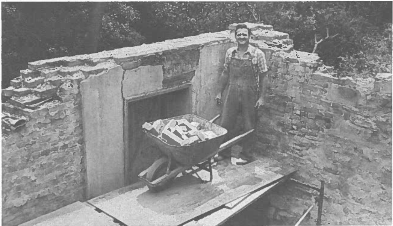
This past spring Don Harbaugh dismantled the brick section of the Fahnestock house. Harbaugh, shown above, estimates that he removed 24,000 bricks by hand from the walls of the house. Renfrew will reuse many of the bricks as it restores the stone section to its original appearance. The bricks not used in the restoration will be available for sale at a cost of 25¢ to 40¢ each. Anyone interested in purchasing Fahnestock house bricks contact Renfrew museum at 762-4723.
