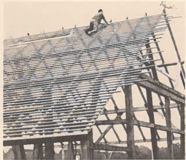
Restoration Craftsman, Terry Pelton, places roofing lathes over the rafters of the Fahnestock Barn.
