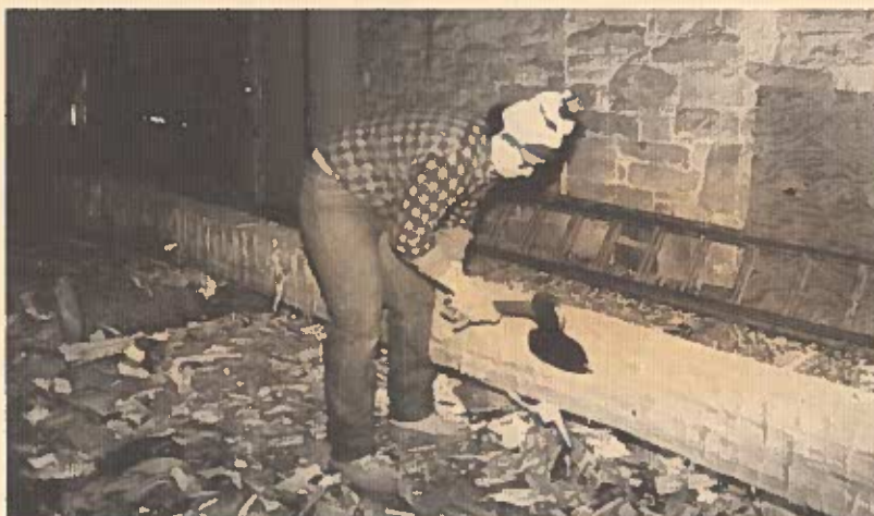
Renfrew's restoration craftsman, Terry Pelton, is shown hewing out a pine timber. Pelton uses a traditional timber framing broad axe to give the faces of the beam a smooth, flat surface. This is 1 of nearly 100 hand-hewed beams that will be incorporated as part of the restoration of the Fahnestock barn.
