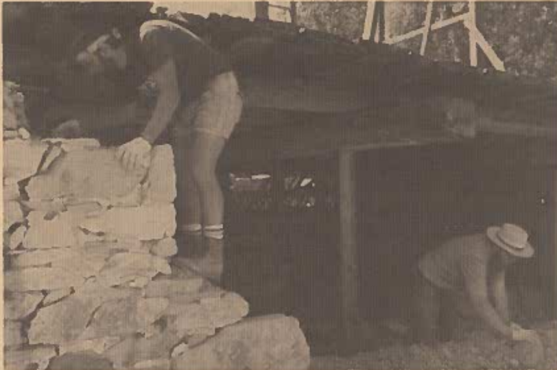
Kenneth Lemmon and Bob North remove the original stonework and mortar (burnt limestone & clay) from the west foundation wall of the Fahnestock barn prior to its restoration. Vegetation and moisture, combined with the weight of the barn's framework, caused the wall to sag outward by more than 1 ft.
